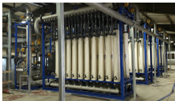
Clifton, Colorado - UF 12 MGD Drinking Water
