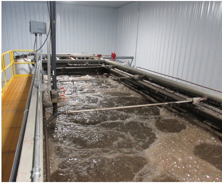
Packaged Plant MBR System at Hamlin Beach WWTP
