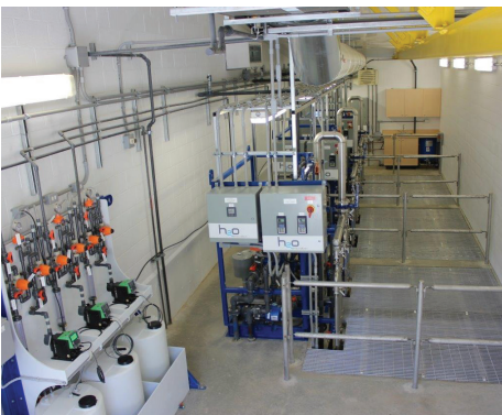
St-Alphonse de Granby - Municipal Wastewater
