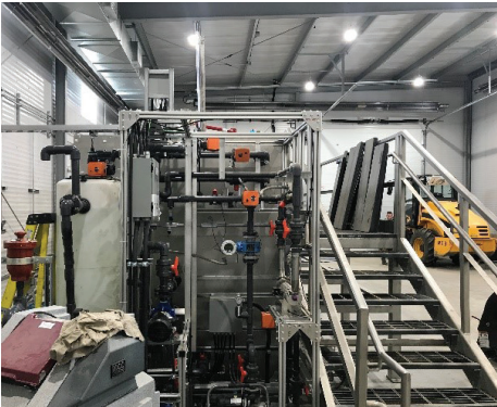
Packaged Plant skids for EMCOR WWTP
