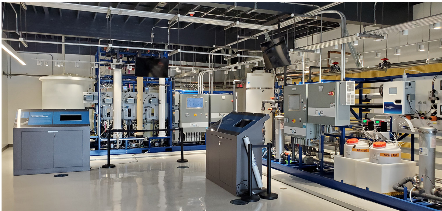
A water reuse and recycling advanced treatment system installed at Las Virgenes Municipal Water District in Calabasas, California.
