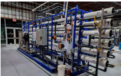
RO Train at Piedmont WaterHub™.
